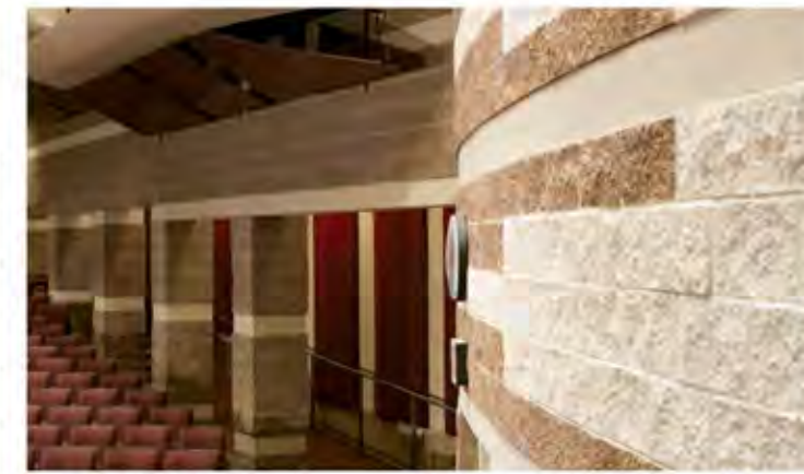
C-TEC – Newark, OH Architect: L. Robert Kimball & Associates Photo courtesy Scott Pease/Pease Photography Colors: Palomino, Vintage
